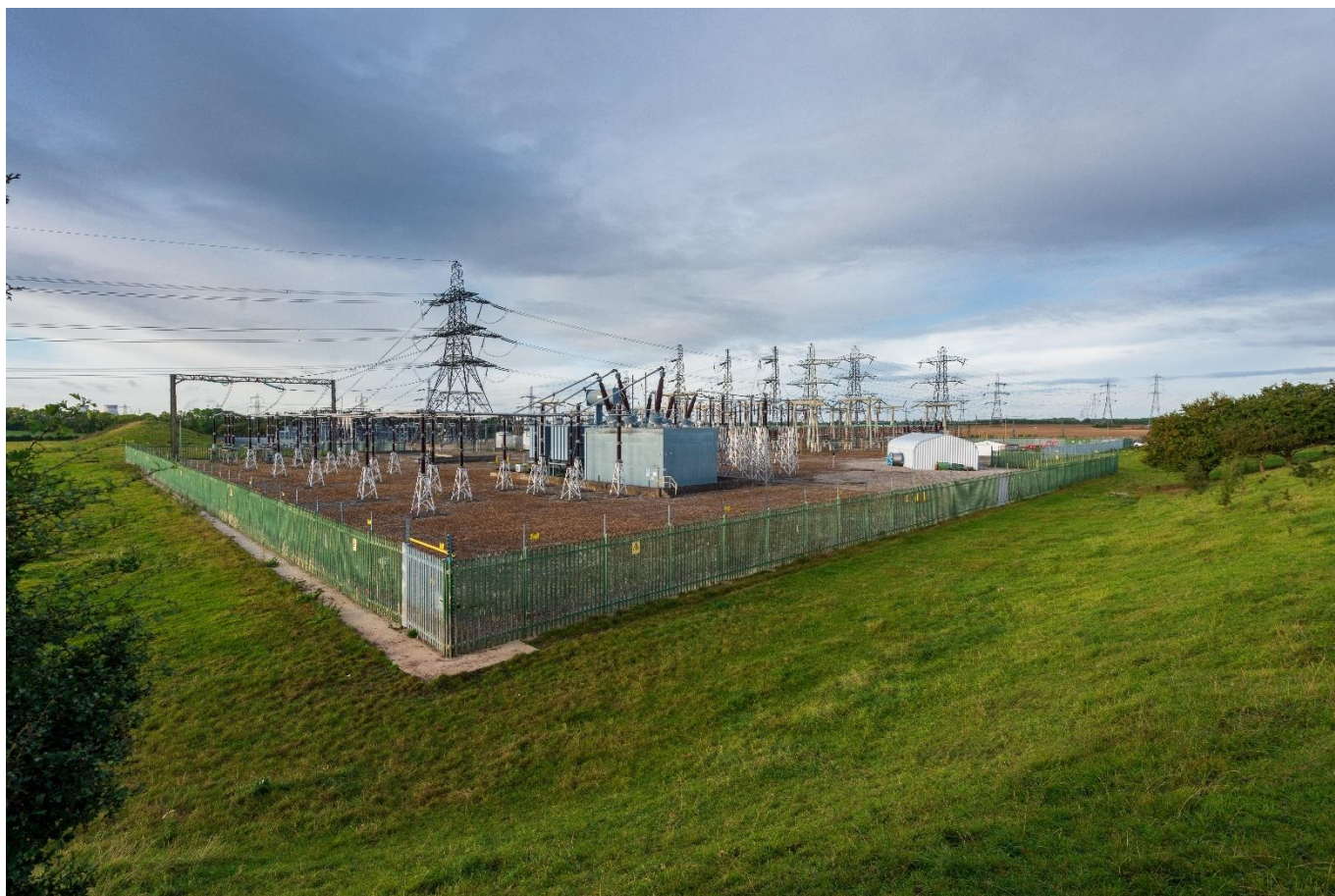
Figure 3.2 – Image of typical substation (existing Monk Fryston Substation)
